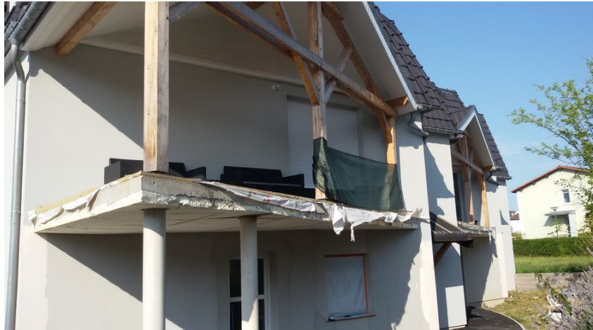
Balcons sans garde-corps
